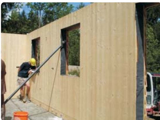
prefabricated BBS-wall with electrical installations, damping and facade
